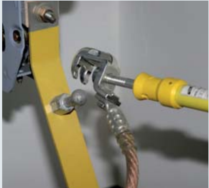
Connecting the phase side of a universal clamp to a fixed ball point.
