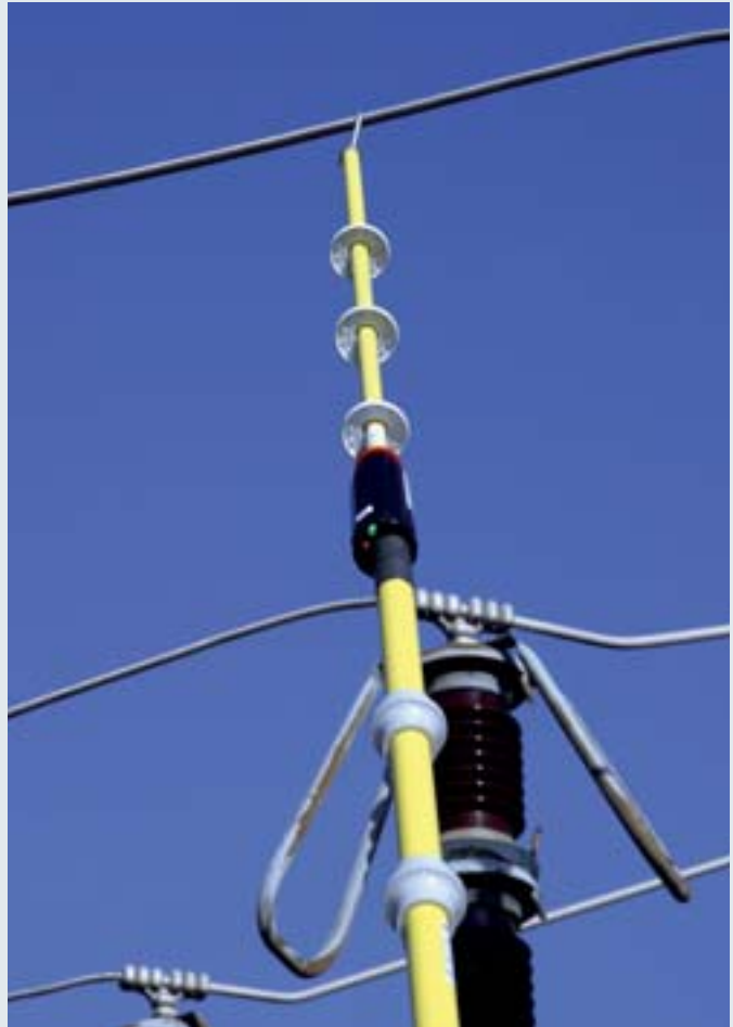
PHE III voltage detector used in an outdoor 110 kV installation.
