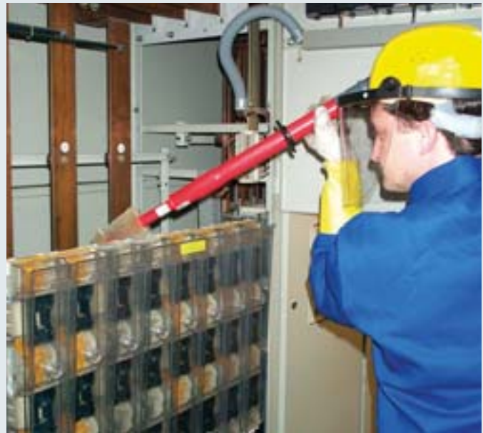
Cleaning a low-voltage switchgear installation under live conditions with TRS NS Dry Cleaning Set
