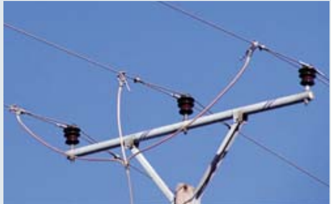
Phase screw clamps used on an overhead line.
