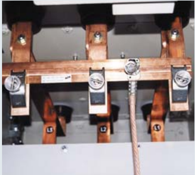
Short-circuiting bar with earthing cable in use in a switchgear installation.
