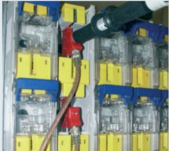
Inserting the fully insulated earthing and short-circuiting device by using earthing handle Type VI.
