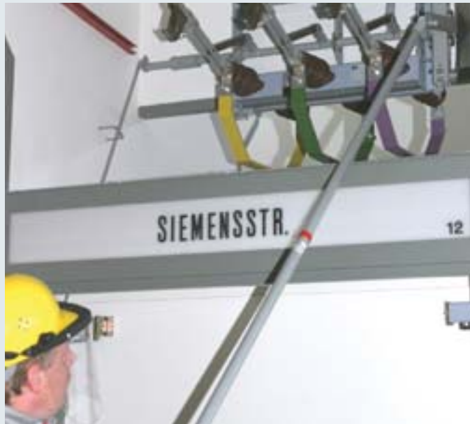
Switching a disconnector with an SCS switching rod.
