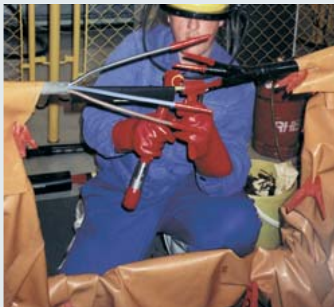
Covering of energised parts.
