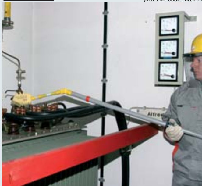
Damp cleaning of a transformer with FRS ZK MS Damp Cleaning Set.
