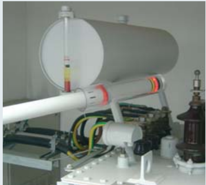
Non-contact voltage detector HSA 205 with attached insulating cap used in a switchgear installation.
