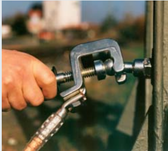
Fixed ball point at a steel tower with mounted universal clamp.
