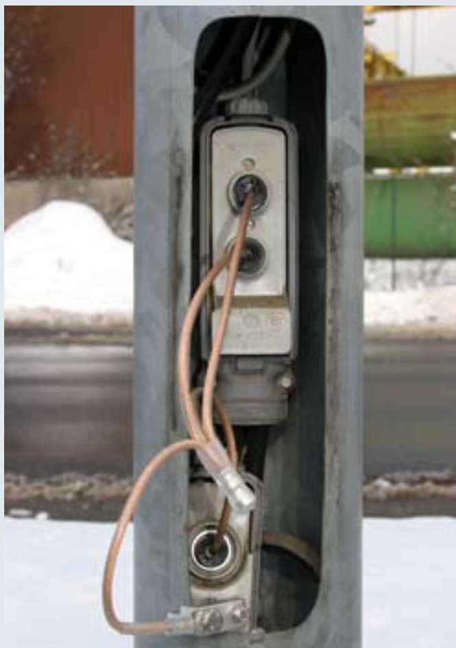
Earthing and short-circuiting device for junction and fuse boxes of street lighting installations.
