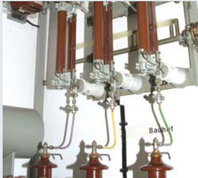
Fixed ball point, attached to the round Cu conductor of a switchgear installation.
