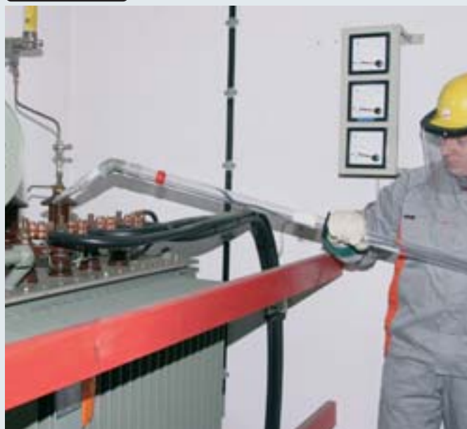
Cleaning a transformer with TRS MS Dry Cleaning Set under live conditions.
