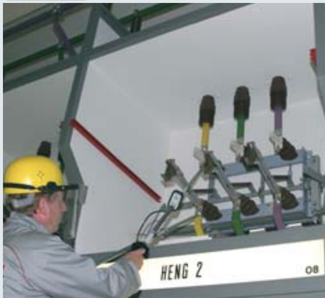
Two-pole PHV phase comparator with green pair of test prods (15 ... 24 kV) used for a 20 kV switchgear installation.
