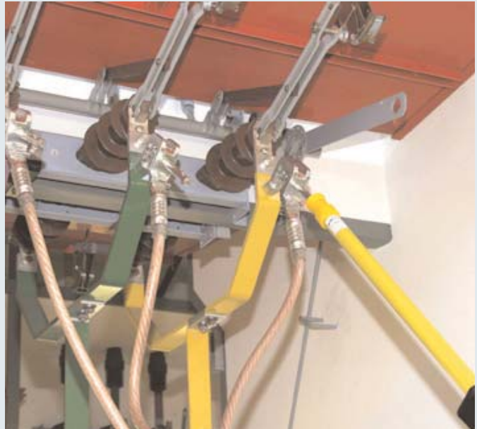
Using an earthing and short-circuiting device with an earthing rod.
