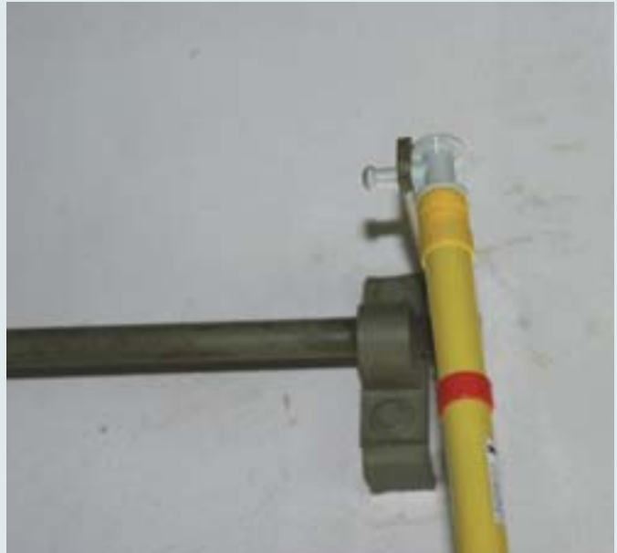
Switching a disconnector by means of an IS SK insulating rod with switching head.
