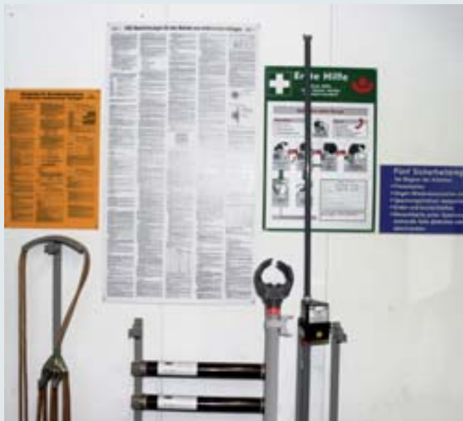
Warning signs displayed at an electrical installation.
