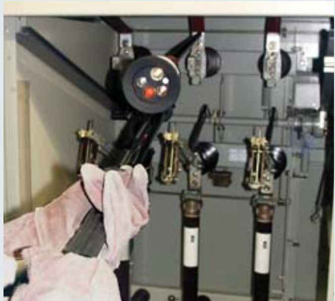
Single-pole phase comparator PHV I used for a switchgear installation.
