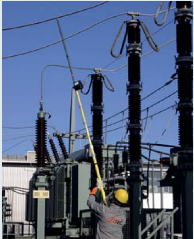
PHE Voltage Detector used in an outdoor installation 110 kV.
